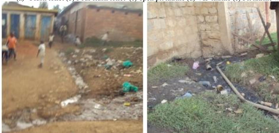
Plate 4: Open drains in Bomet municipality
